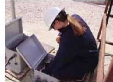
On site, a technician hooks up to the system via laptop to analyze error codes.
